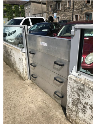
Flood protection blocks access
