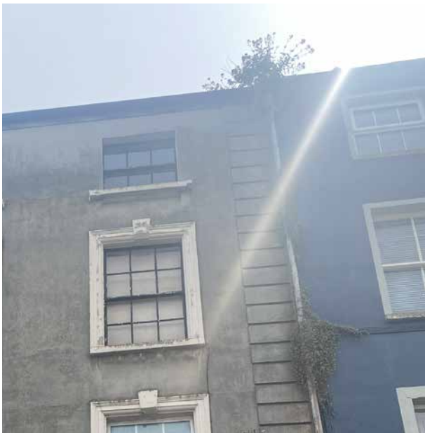
Figure 90 - Vegetative growth adjacent to inadequate rainwater goods
