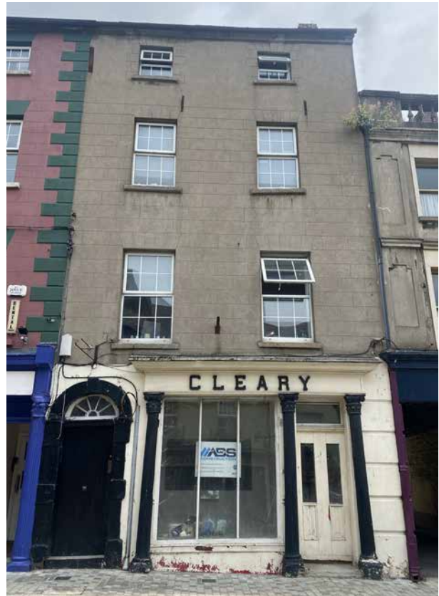
Figure 61 - Lack of maintenance and repair and uPVC windows
