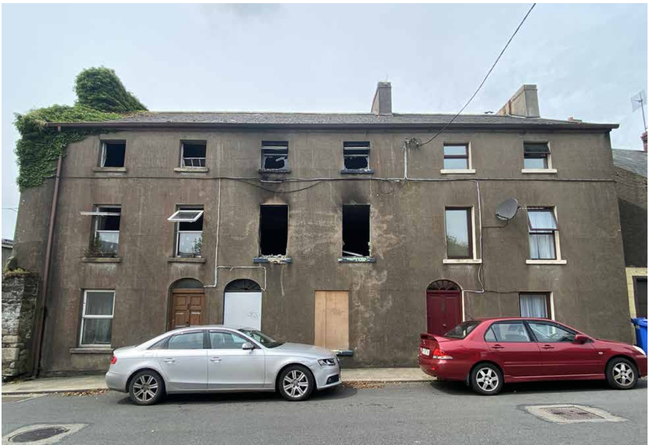
Figure 48 - Burnt out houses
