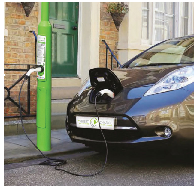
Charging incorporated in to light columns
