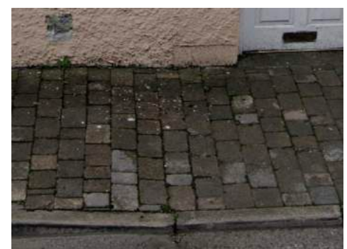
Pavement at Henry Street
