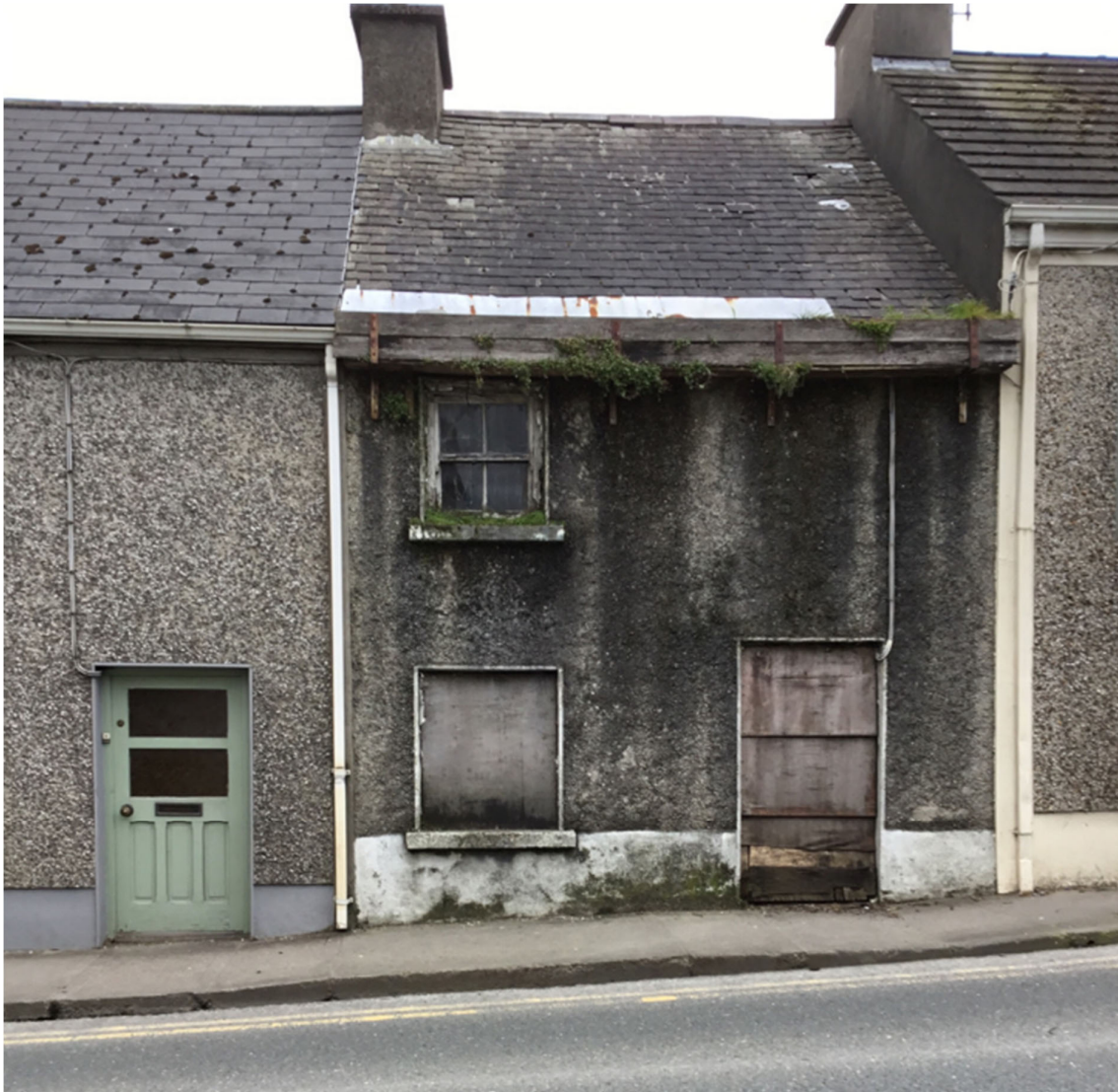
Figure 5-10: Derelict Residential Building on Limerick Street.
