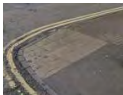
Figure 91 - Pavement at Thomas Street
