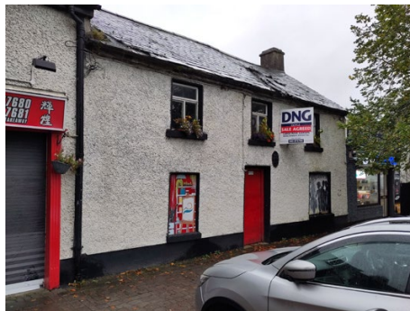
Existing vacant development along Main Street to be retained and enhanced with the potential to open up access to backlands.
