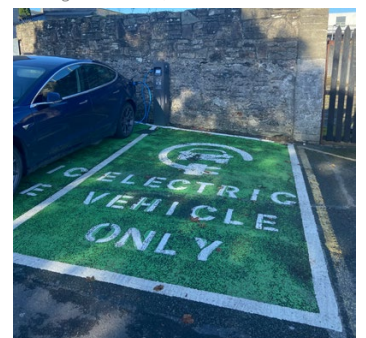
Electric car charging point, Main Street Car Park
