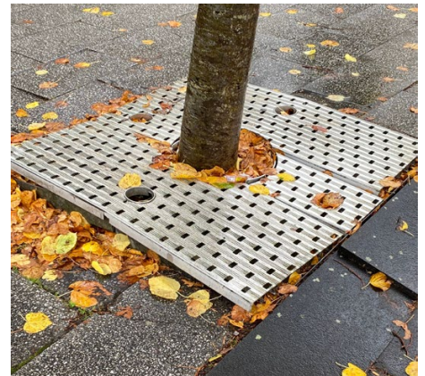
Existing trees along Newtown Square showing signs of tree root egress which is lifting the paving within the canopy diameter of the tree. Some areas of paving have become a trip hazard as a result.
