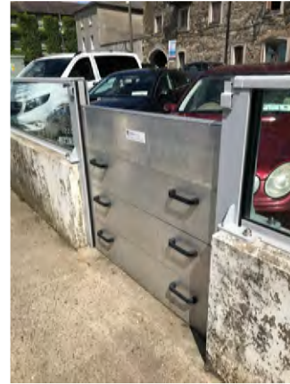
Flood protection blocks access
