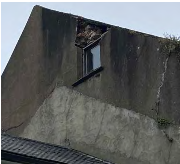
Figure 62 - Poor maintenance, Quay Street
