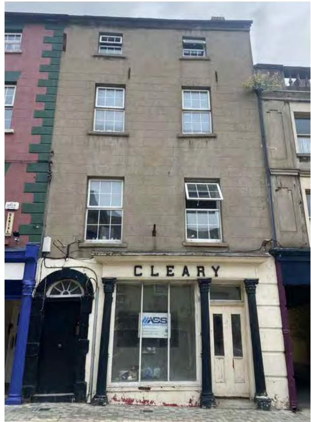
Figure 60 - Lack of maintenance and repair and uPVC windows
