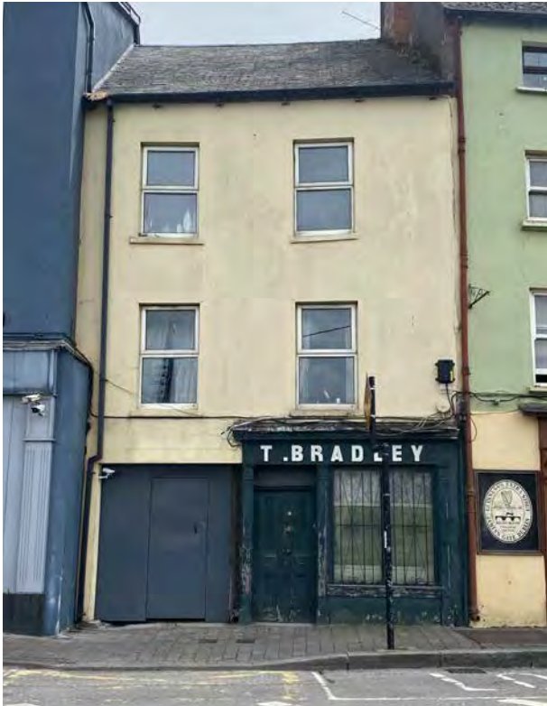
Figure 88 - Subsidence evident, The Quay
