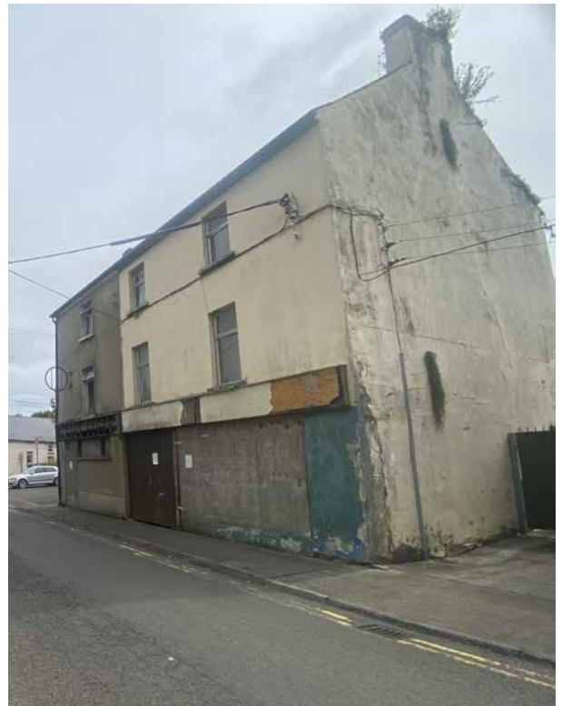
Figure 43 - Derelict building, Priory Street
