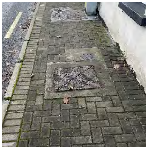
Poor quality surface finishes
