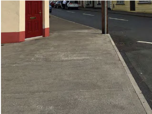
In situ concrete concrete paving denotes low quality, with pole at the kerb edge which limits useable space and is dangerous for vehicles
