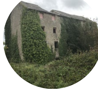
One of the old Grain Stores which requires urgent repair
