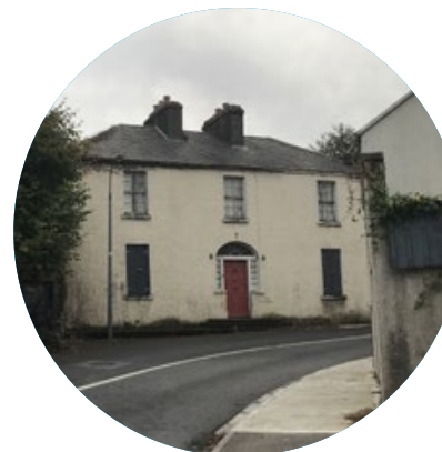
The Old Deanery to the south of Barrack St beginning to show signs of significant decay
